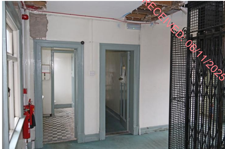
Plate 21: Landing at lift cage
